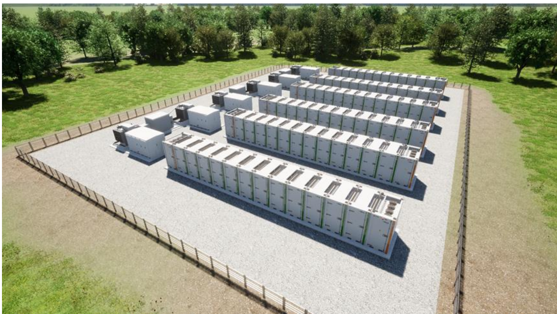
Image 4.6 Typical BESS Units
