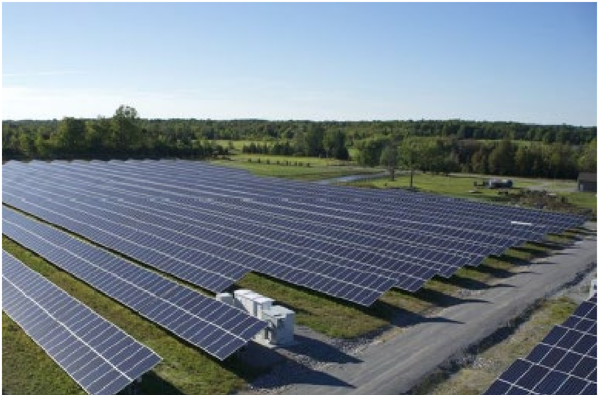
Image 5.1 Typical Fixed PV Arrays (with Conversion Unit)
