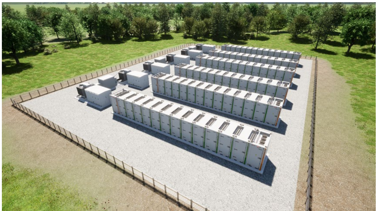
Image 5.6 Typical BESS Units
