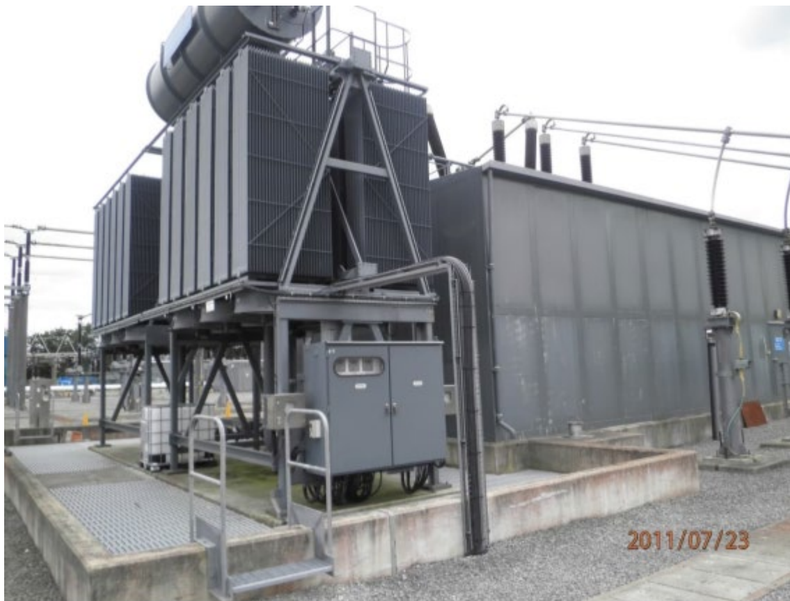
Image 5.5 Air Insulated Substation
