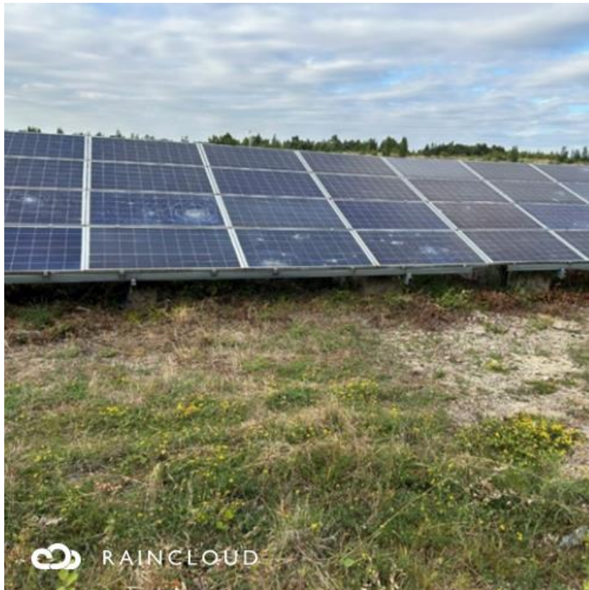
Image 12.6 and Image 12.7 Vandalised PV Arrays, Thorne Solar Farm, Doncaster (2024)
